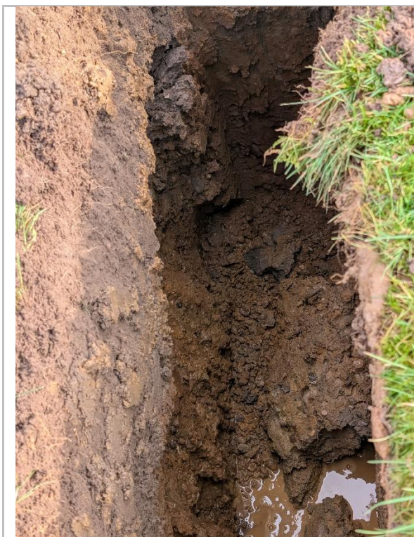
Figure 17. Initial Side Wall Collapses (TP102)
